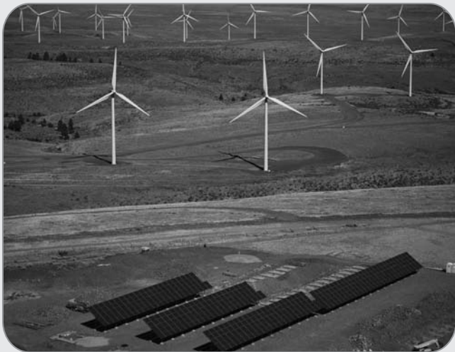
A solar-power generating plant operates alongside the 127 turbines at PSE's Wild Horse Wind and Solar Facility in Kittitas County.
