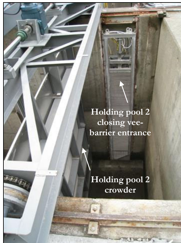
Figure 9. Closing vee-notch weir located between holding pools 1 and 2.
