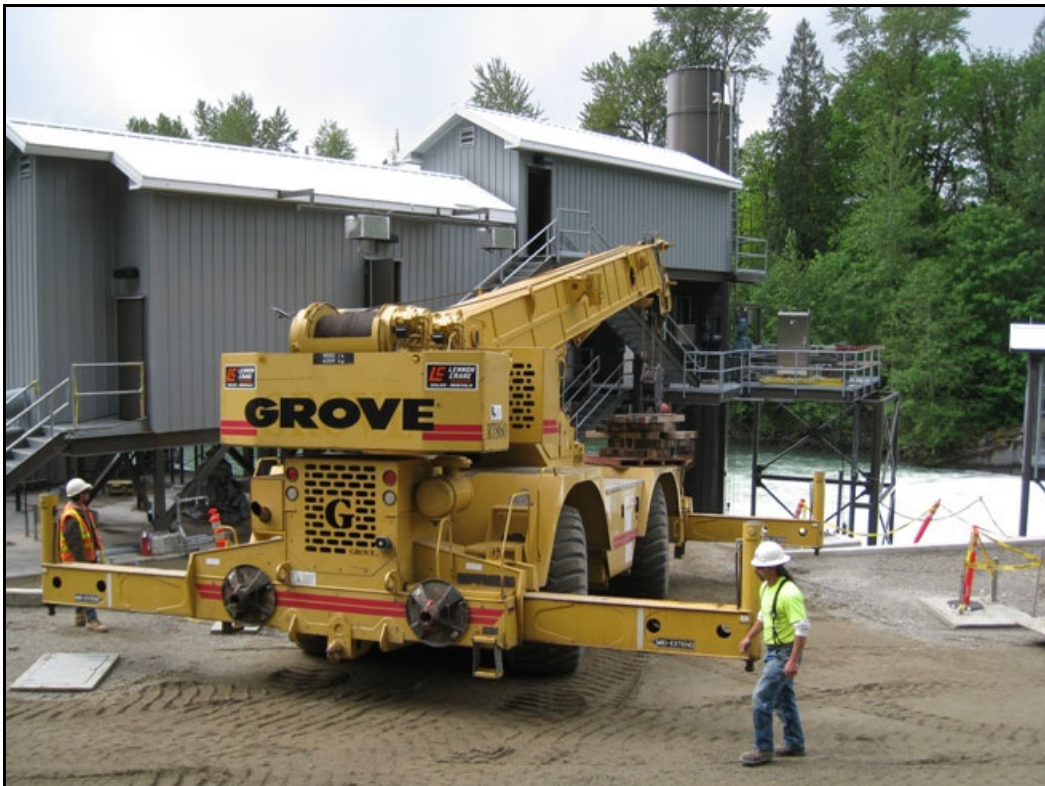
Figure 23. Grove RT-860 portable crane positioned to lift fish during emergency fish evacuation.
