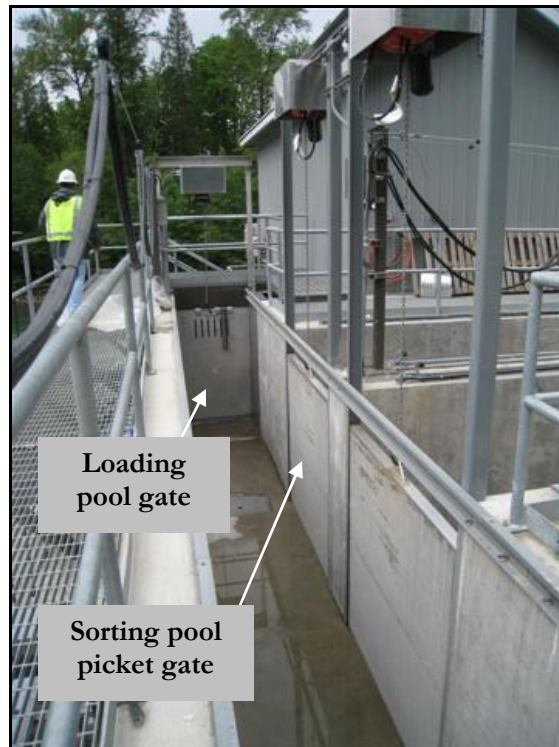
Figure 18. Loading pool gate.
