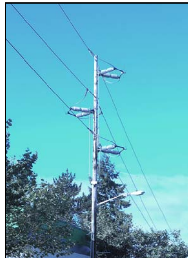
Example of a transmission switch
