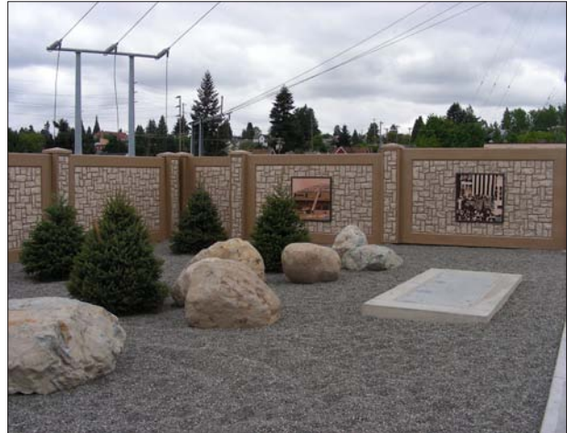
Architectural wall surrounding Bremerton substation
