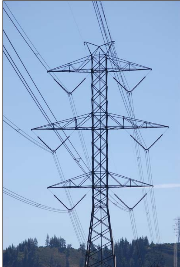
PSE’s transmission and distribution systems are already highly automated, with sensors that monitor the electrical grid every four seconds.
