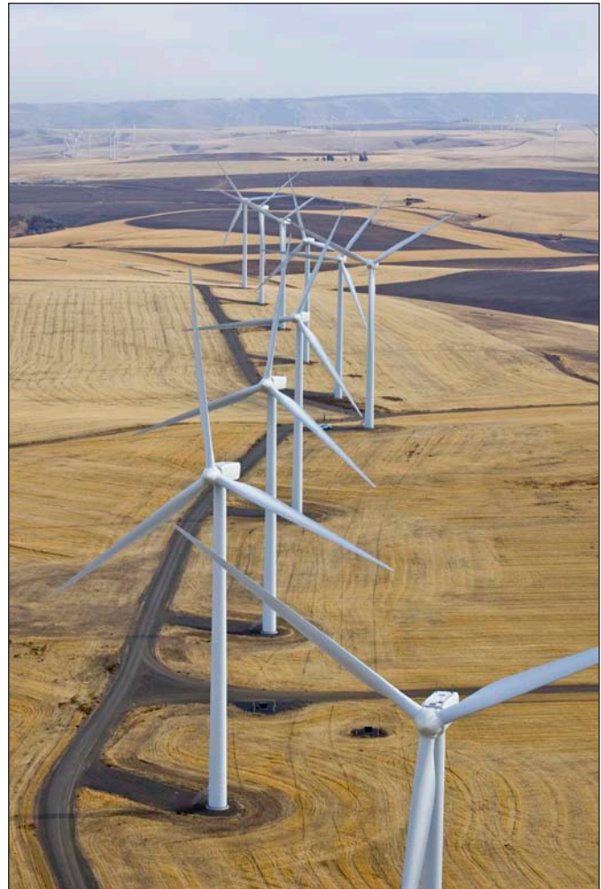
PSE is a leader in owning and operating wind power, with generating capacity equal to the electrical needs of approximately 100,000 homes.
