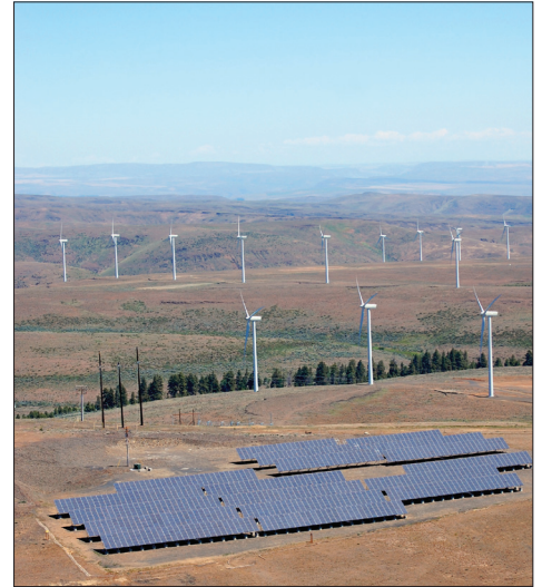
At 500 kW, the Wild Horse solar array is the Northwest's largest demonstration project of photovoltaic technology, which turns sunlight into electricity.
