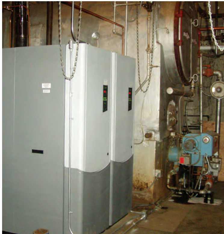
PSE incentives covered over half the installed project cost of the boiler upgrade shown here.
