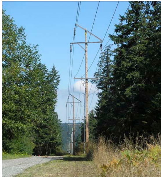
Transmission lines on Whidbey Island
