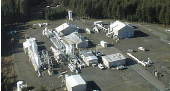
One-fourth of the natural gas Pacific Northwest homes and businesses require on a cold winter day can be drawn from Puget Sound Energy's newly expanded Jackson Prairie gas-storage facility in Lewis County.
