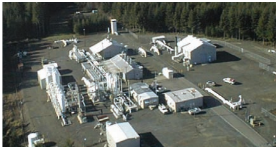
One-fourth of the natural gas Pacific Northwest homes and businesses require on a cold winter day can be drawn from Puget Sound Energy's newly expanded Jackson Prairie gas-storage facility in Lewis County.
