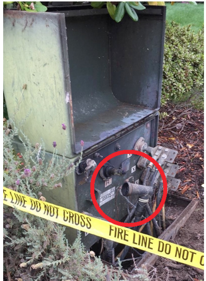
Transformer with lid open, exposing an energized 7.2kV elbow.
