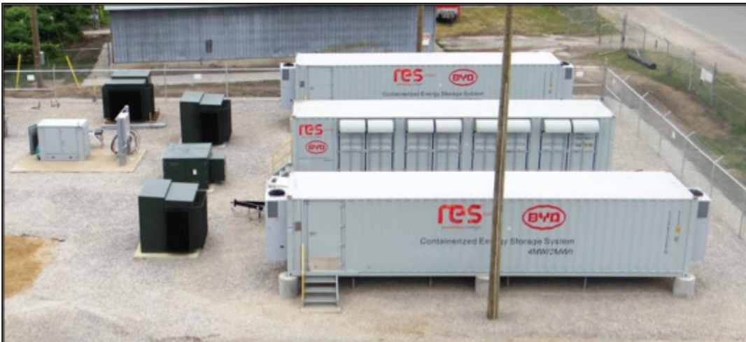
4 MW/2 MWh distribution-connected lithium-ion battery
