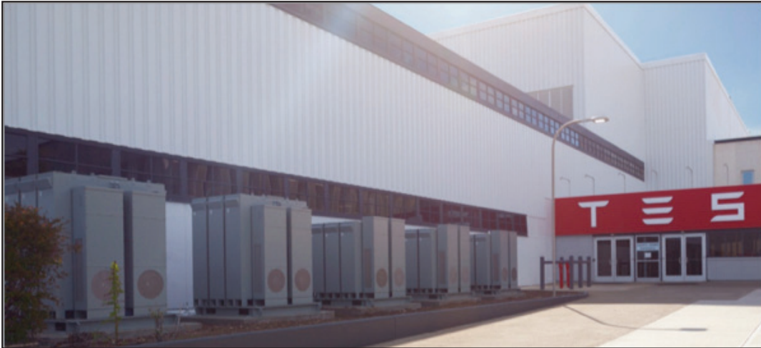
1 MW/2 MWh customer-sited lithium-ion battery.
