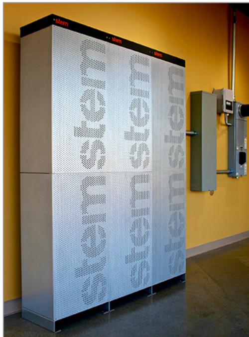
54 kW/54 kWh customer-sited lithium-ion battery.
