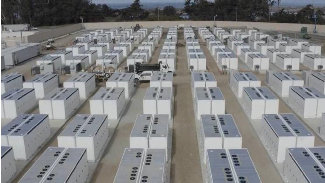
Source: PG&E; Moss Landing Battery Energy Storage
