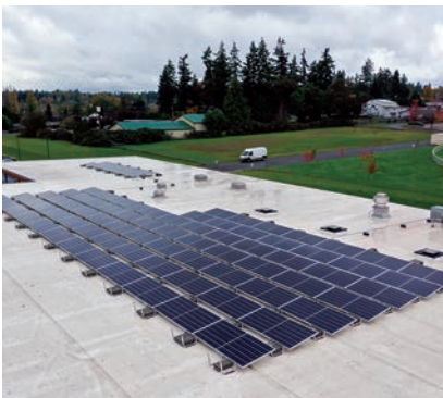
Solar installation at the Boys & Girls Club of South Puget Sound Bremerton
