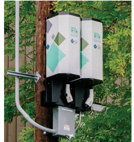
Port Orchard EV pole charger
