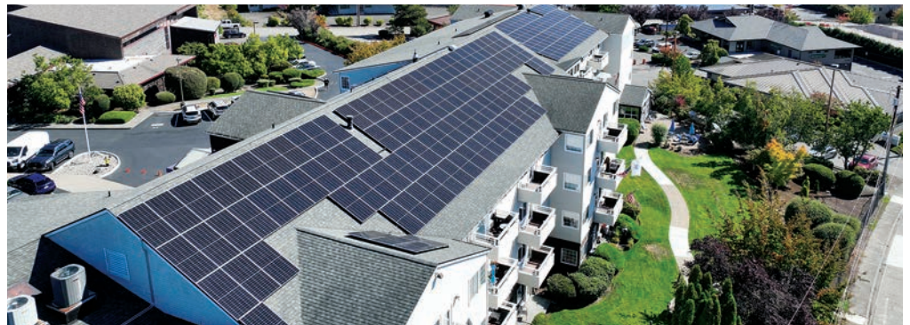
Solar installation at Canterbury Manor, a senior living community in Bremerton
