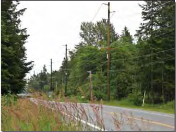
Single-circuit 115 kV wood pole with distribution underbuild
