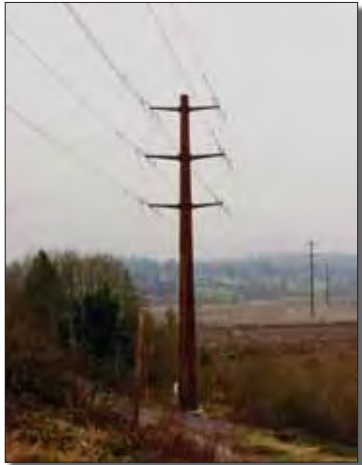
Double-circuit weathered steel monopole
