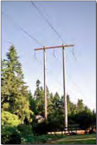
Single-circuit 115 kV wood H-frame structure
