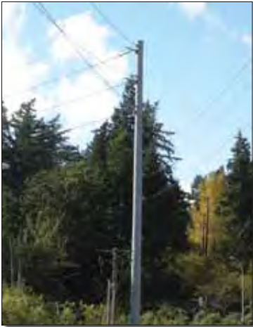
Single-circuit galvanized steel monopole
