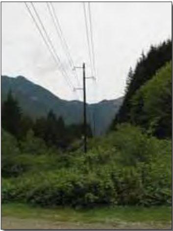
Single-circuit 115 kV wood pole with bundled conductor
