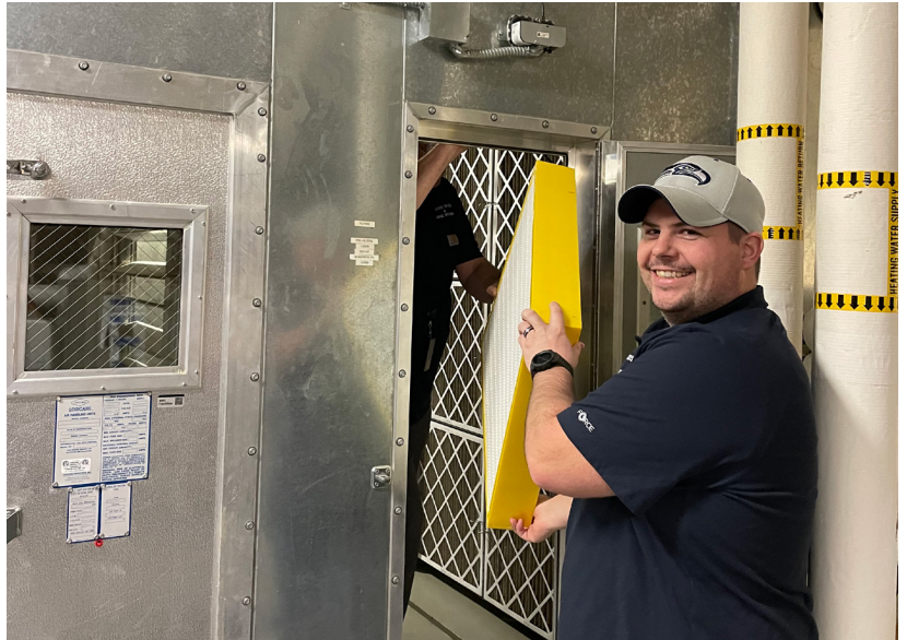
The Accelerator emphasizes the significance of regularly replacing HVAC filters to prevent pollutant overload and improve energy performance.
