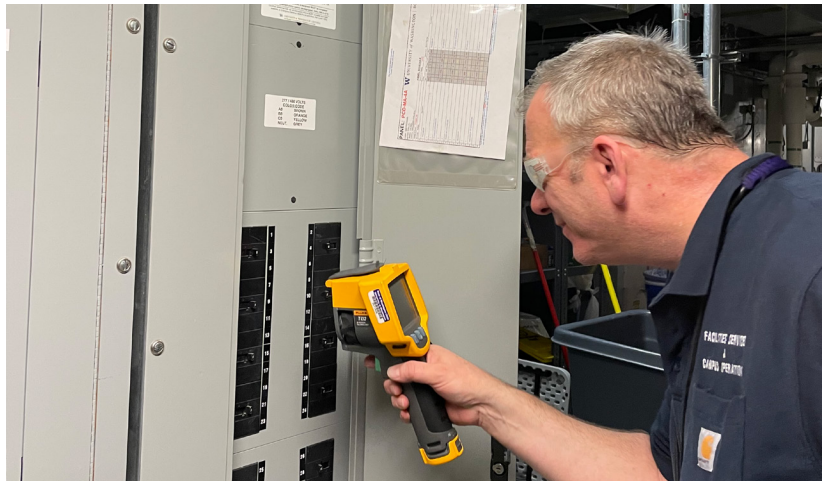
UW Bothell learned the importance of regular energy audits in the Accelerator. They include checking the temperature of circuit breaker panels, which helps detect deficiencies that may increase energy usage and potentially disrupt service.
