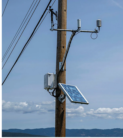
Weather stations collect more granular and localized data
