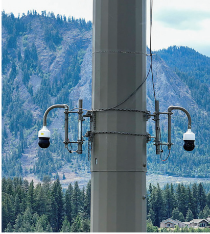
Pano AI smoke-detecting cameras aid in fire response on suppression.
