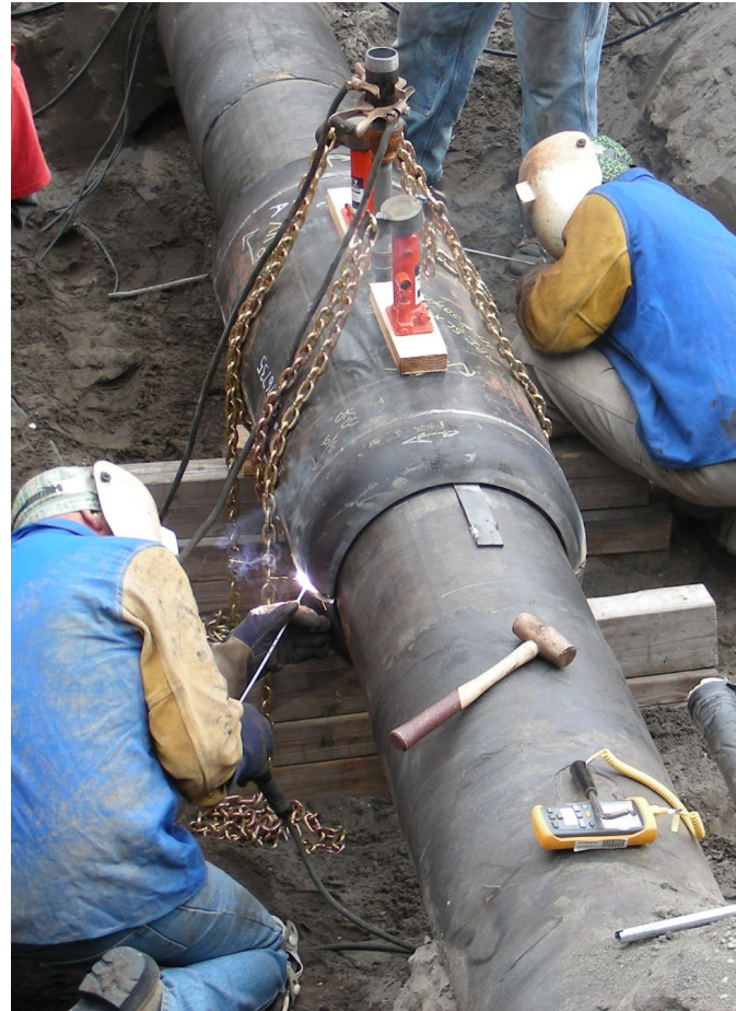
Certified pipeline welders working on repairs to a PSE pipeline in Seattle.
